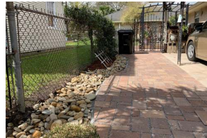
Newly installed infiltration trench and pervious pavement, designed to reduce standing water during rain events - GENTILLY
