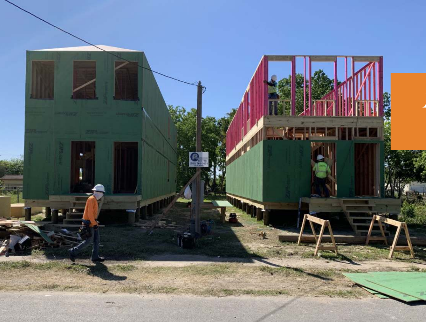
Affordable residential construction as part of the Lower Ninth Ward Development Initiative - LOWER NINTH WARD
