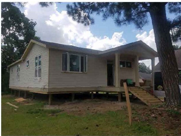
First O-HIP home developed by Home by Hand is under construction in Gentilly.
